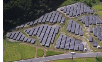
Off-site PPA solar power generation equipment (partial)
